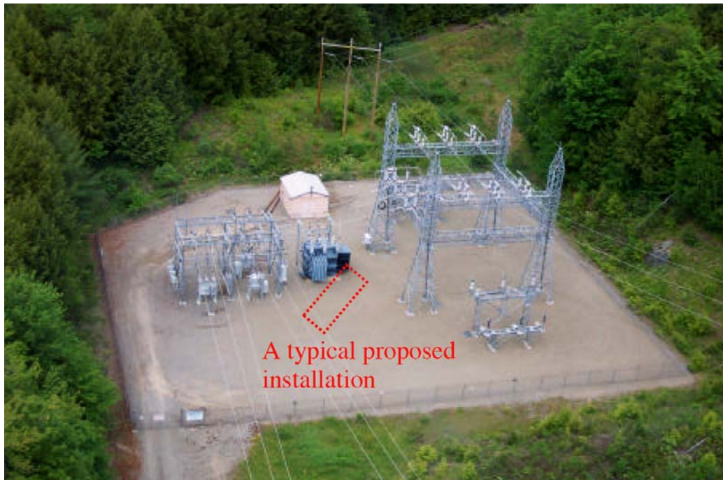
Fig. 10. MTS proposed position within Vermont Electric substation.
